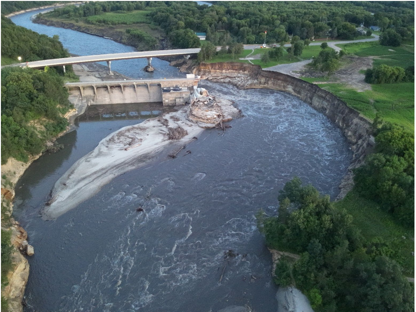
Figure 5 Rapidan Dam west abutment breached following June 2024 historic rain (Photo Credit: Blue Earth County Sheriff's Office)
