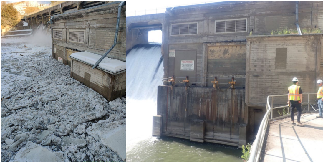
Figure 4 Comparison: Downstream ice buildup (left), January 18, 2020 (note white signs on powerhouse for scale of ice dam height) vs. normal tail water (right) [Photo Credit: Blue Earth County (left), Barr Engineering Co. (right)]
