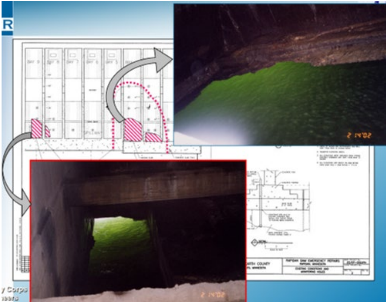
Figure 3 Voids in concrete base that should be founded on bedrock (Photo Credit: Barr Engineering Co.)
